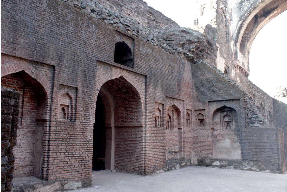
Plate 4: Dar-us-Shifa at Mandu, Lakhori brick work used for repairs, Photo taken by the author
